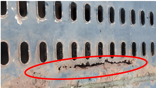
Figure 1A: oxidation passing through the decking
